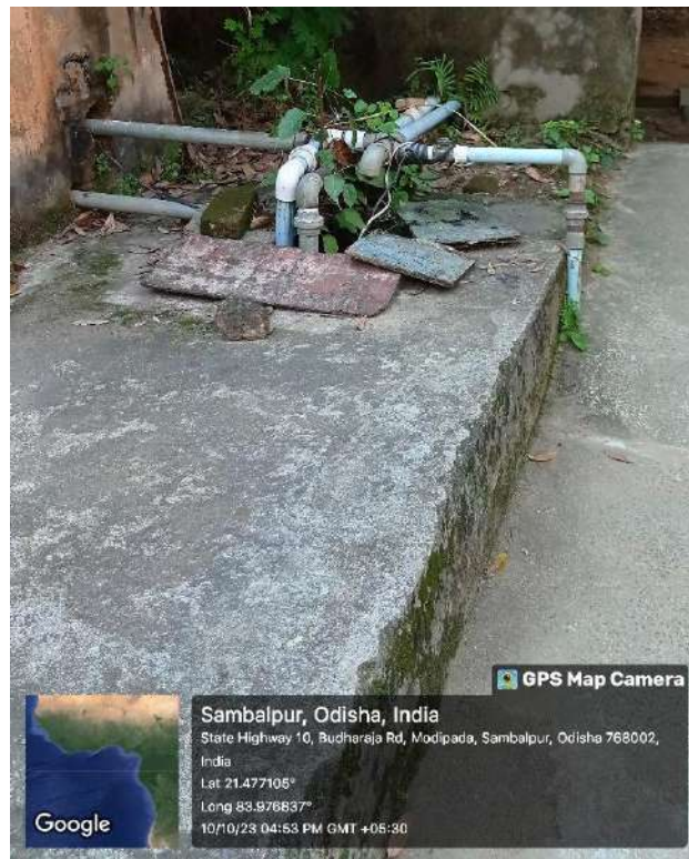
Pumping System at G.M. University
